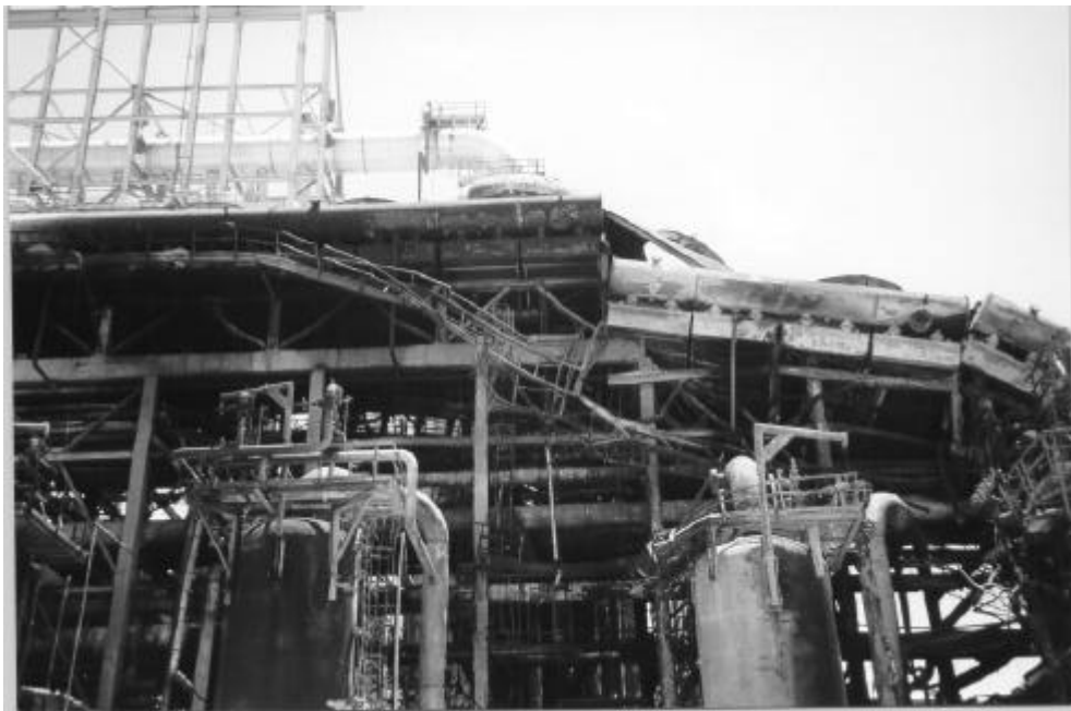
Figure E-4: Photograph of explosion and fire damage at OP-III as seen from north side of pipe rack, looking upward.
