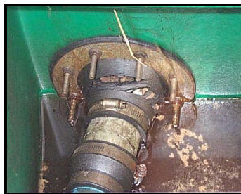
Sump penetration seals in poor condition
