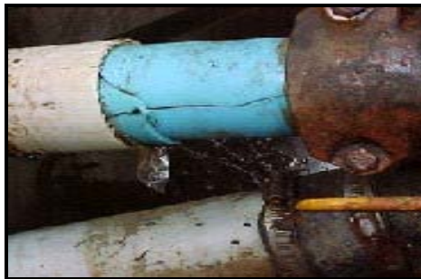
Flexible piping is cracked
