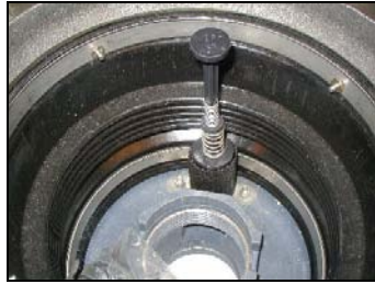
Spill bucket drain valve
