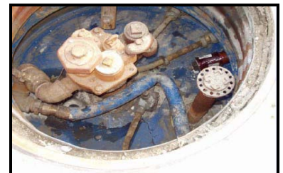
Flexible piping is kinked
