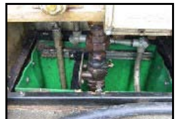
Contained dispenser sump
