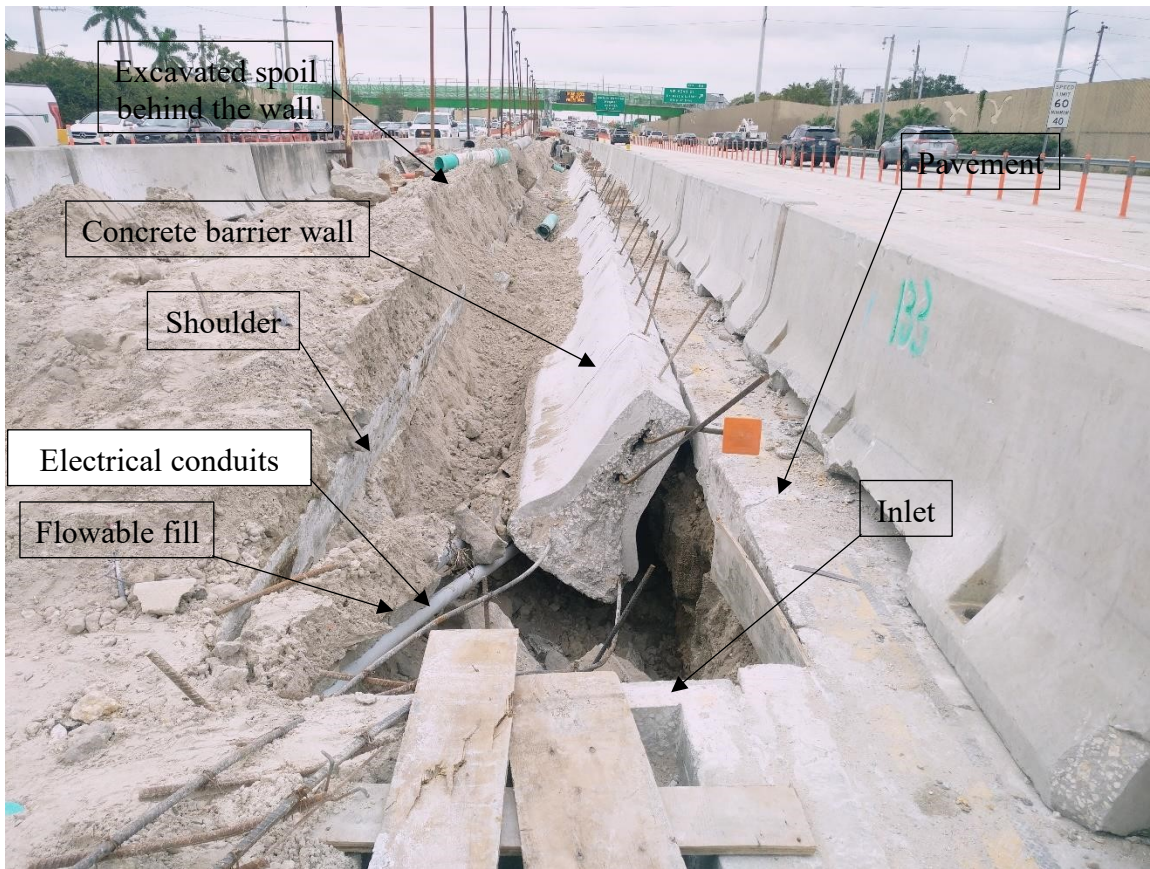
Figure 5 Scene of incident – looking south (North end of the barrier wall)
