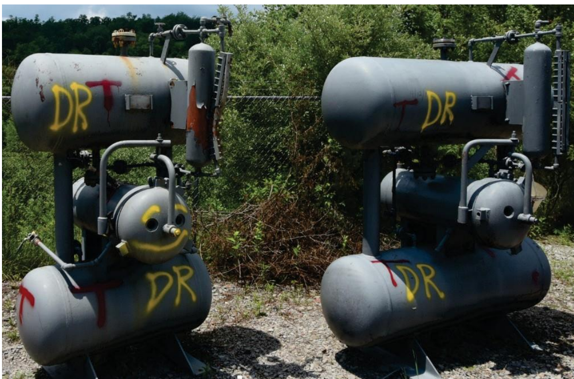
Figure 8. Drained Status. This photo shows how MRR technicians spray painted odorizer equipment with a “D” or a “DR” for drained (in yellow) after they drained the sodium hypochlorite treatment solution from the odorization equipment. (Credit: CSB).
