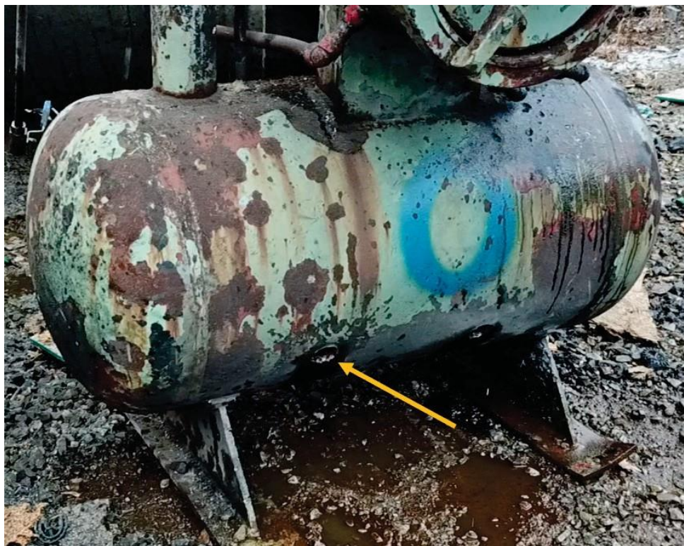
Figure 20. Drain Hole. This drone image shows one of the holes cut by the explosion venting process used to drain the bottom chamber of an MP vessel. (Credit: MRR).
