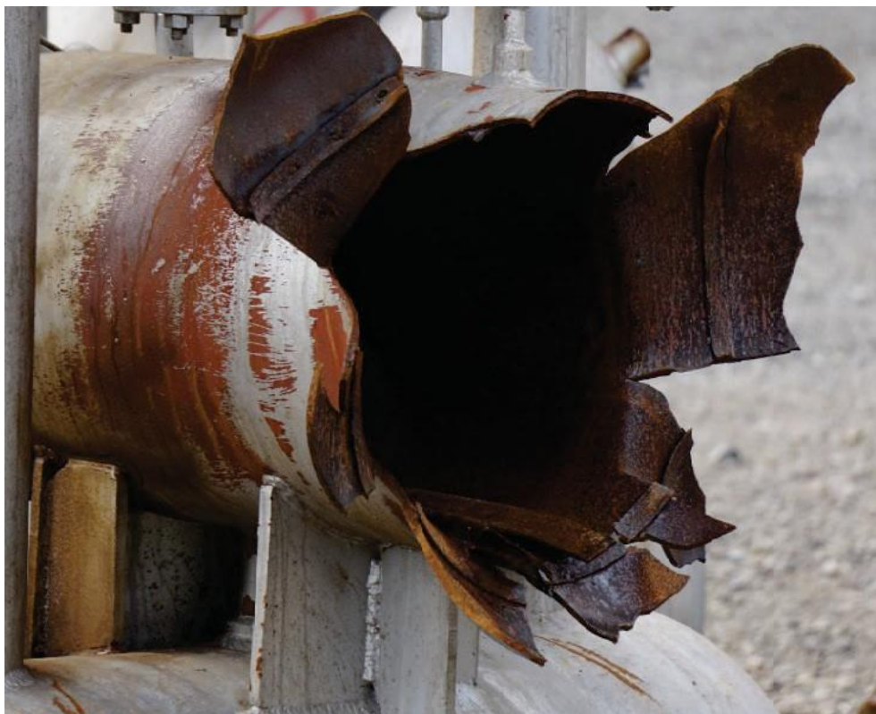
Figure 17. Ruptured MP Odorizer Middle Chamber from June 20, 2017, Incident. This photo shows the post-incident condition of the rounded end of the middle chamber that ruptured in the June 20, 2017, explosion. (Credit: SPSI).
