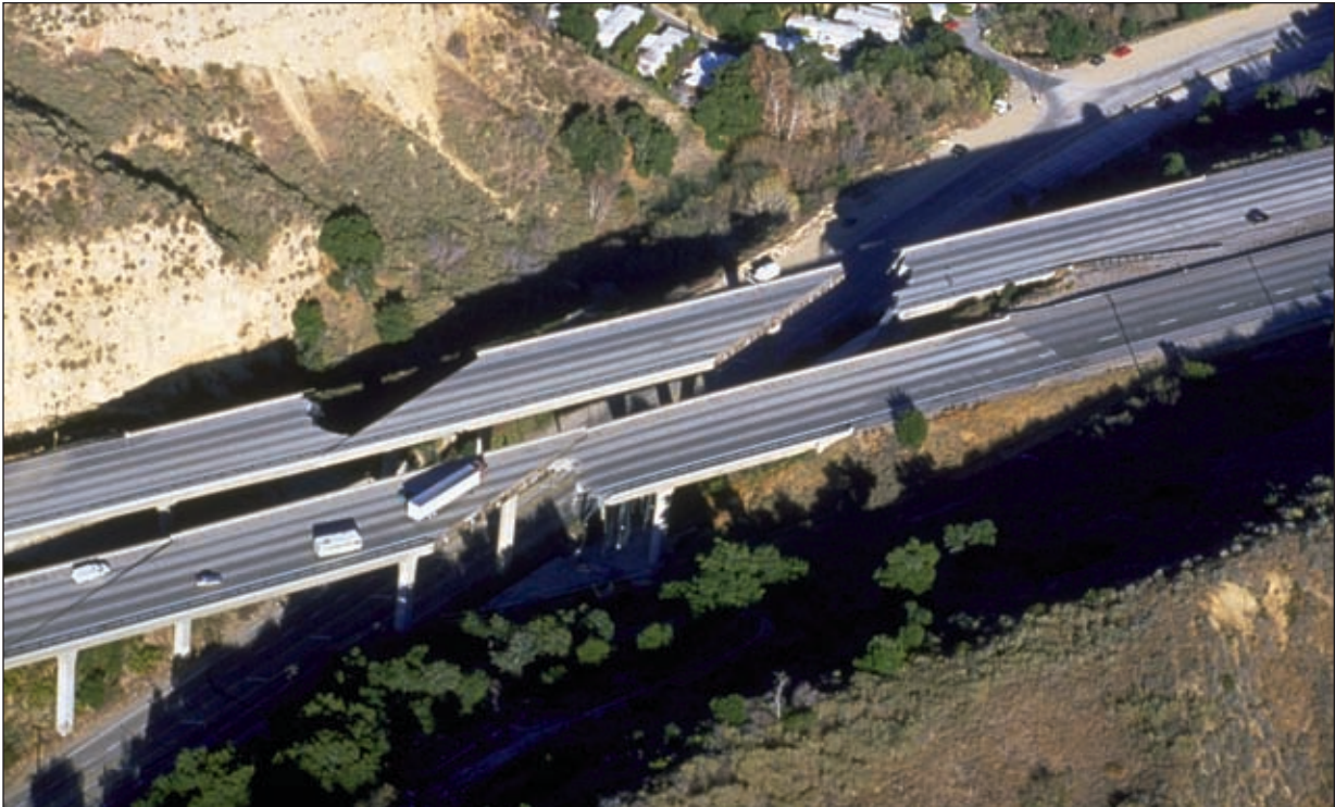
Northridge Earthquake, CA, January 17, 1994 – Many roads, including bridges and elevated highways, were damaged by the 6.7 magnitude earthquake.
