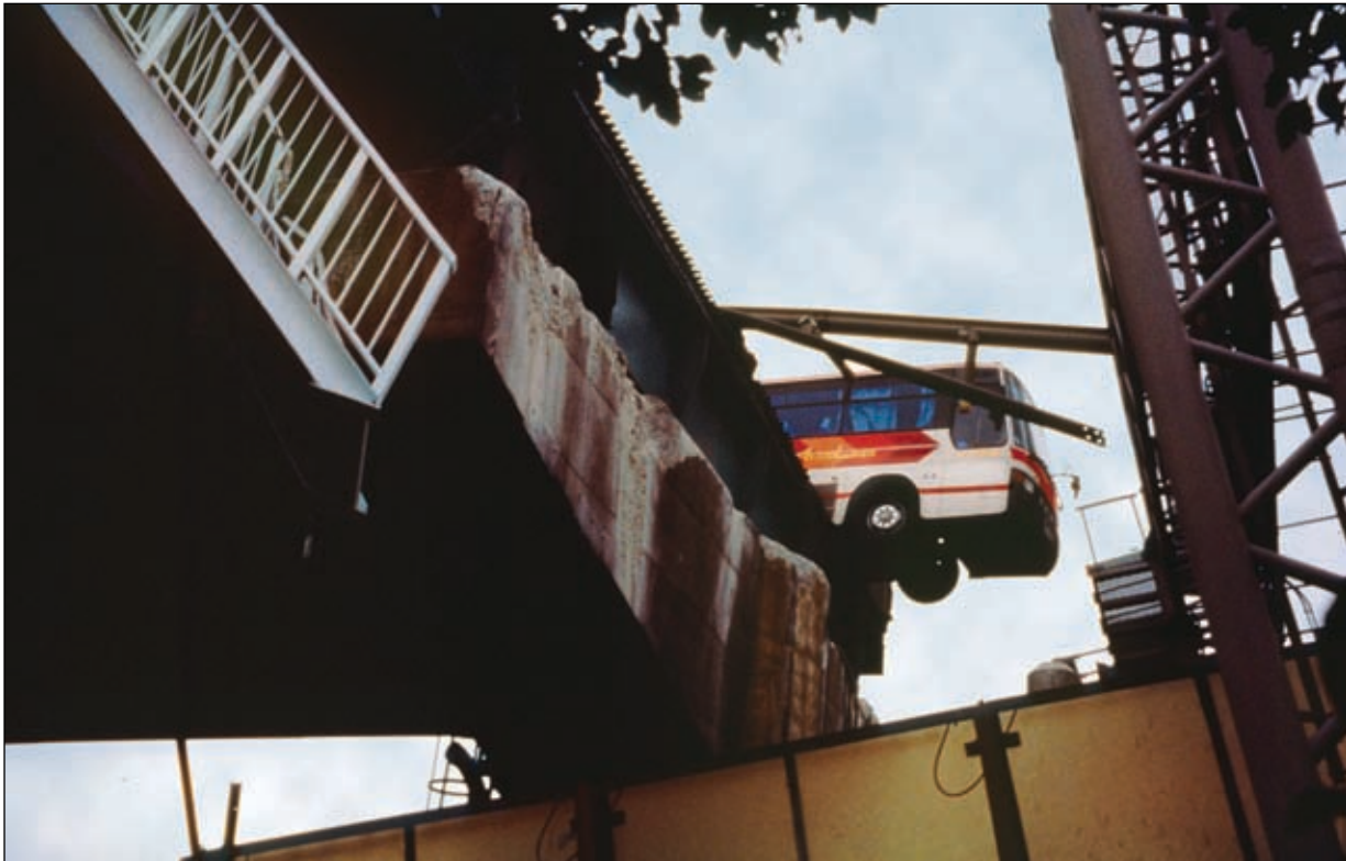
Kobe Earthquake, Japan, January 17, 1995 – A bus filled with holiday skiers stopped just short of disaster on a damaged section of the Hanshin expressway. (Copyright 1997 by Earthquake Engineering Research Institute)
