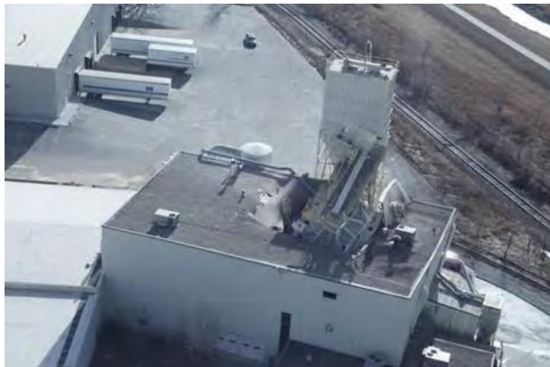
Fig. 2 Aerial view of collapse
