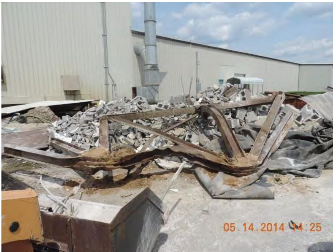
Fig. 107 Exterior truss after being retrieved
