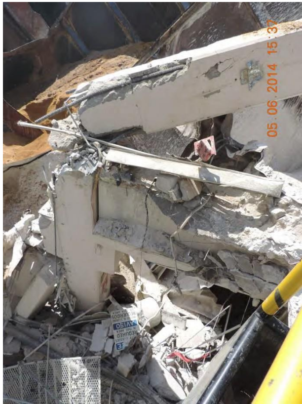
Fig. 100 Fracture of NE corner column at 3 rd floor
