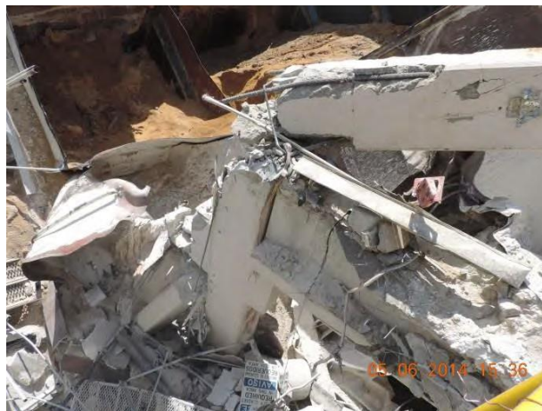
Fig. 101 Another view of fracture of NE column at 3 rd floor
