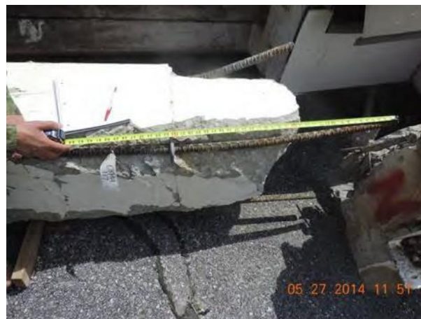
Fig. 103 NE corner column showing inadequate lap splice
