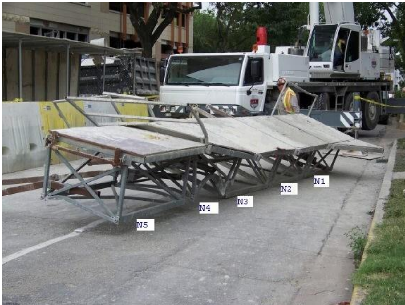
Figure 2 - Failed Deck Modules (North side)
