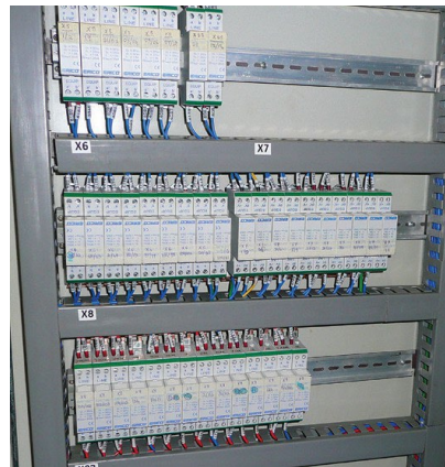
Figure 114. Industrial facilities may require many circuits to be protected.
