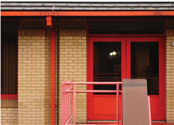
Figure 54. Example of poorly located a down-conductor.
