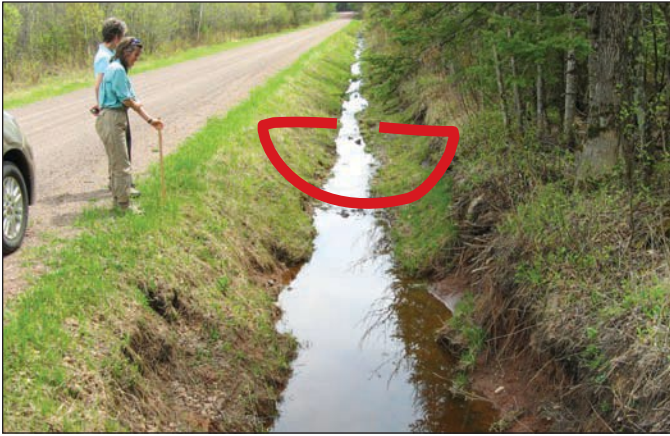
Figure 37: Ditch with vertical back slope sloughing due to instability
