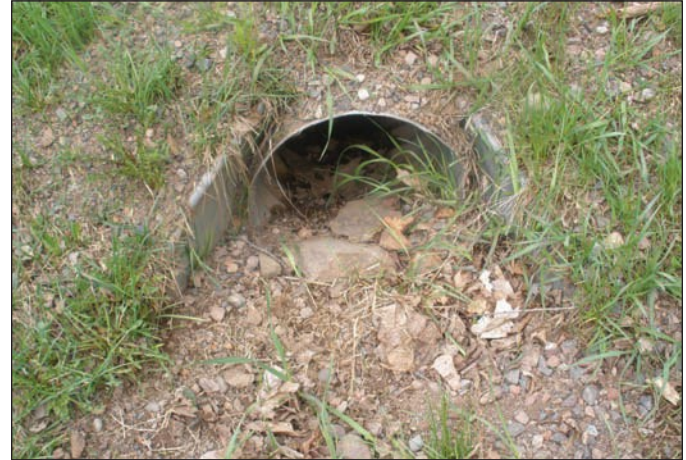
Figure 4: Debris blocking culvert
