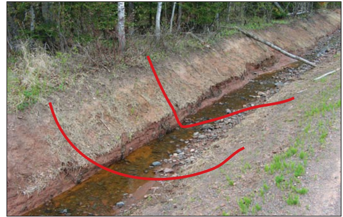
Figure 38: Rounded-bottom ditch incising toward a V shape after heavy rainstorm
