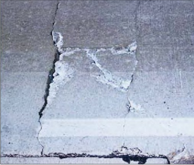
Figure 7. A typical CRCP punchout distress.
