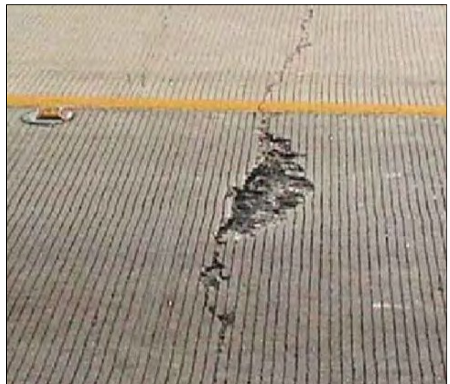
Figure 9. Spalling along transverse crack in a CRCP.
