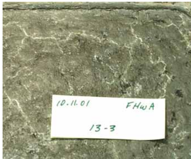
Figure 16. Cracked curing membrane resulting from application before cessation of bleeding.
