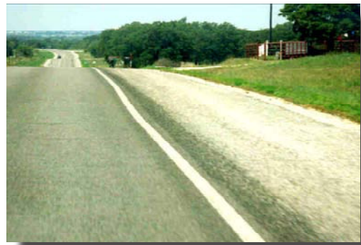
In addition to paving the shoulder, color variation between the shoulder and travel lanes adds visual delineation.
