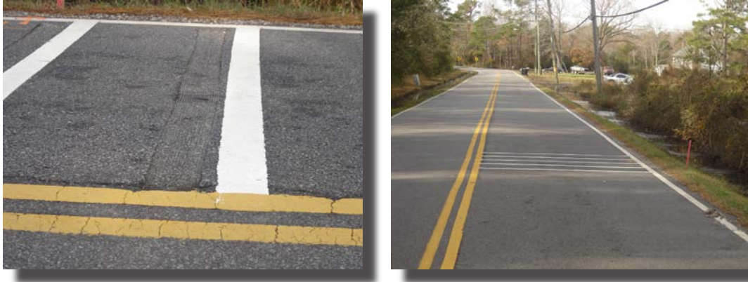
For this RRS application a set of 5 grooves and painted lines were placed 200 ft before the curve.
