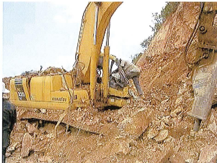
Figure 6. Location of the Komatsu PC 220 Excavator during the Rescue Operation, Looking Toward South (Provided by GEC, LLC.).
