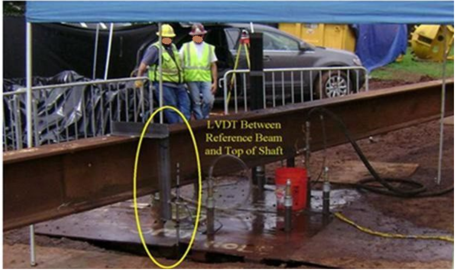
Figure 6.2: Photograph of an LVDT between the reference beam and the top of the shaft during grouting (courtesy of Applied Foundation Testing).
