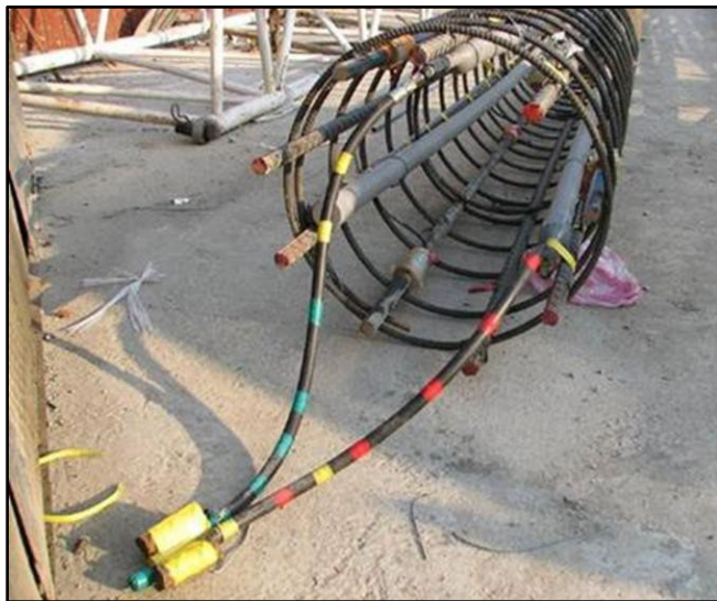
Figure 5.6: Photograph of a sleeve-port system constructed using flexible hoses (courtesy of Dr. H.H. Hsieh).
