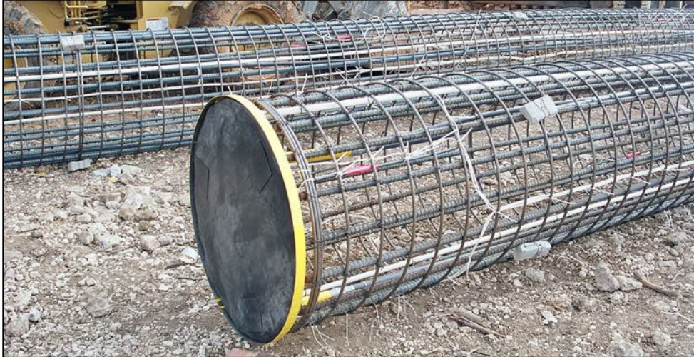
Figure 5.9: Flat-jack post-grouting device on a 4-ft diameter shaft (photo courtesy of Applied Foundation Testing).
