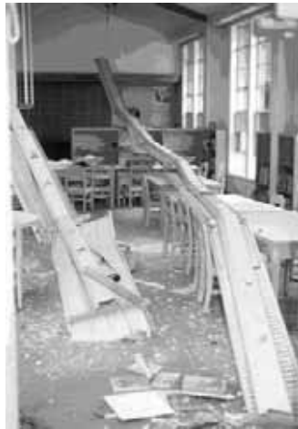
Figure 9-5: Falling objects can be a direct threat to life, as can be envisioned in this example, had children been sitting in the seats in this elementary school library in Coalinga in 1983.
