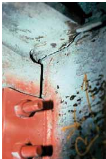
Figure 6-7: Northridge, 1994 Failure of a welded steel connection.
