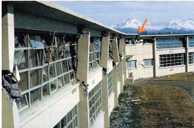
Figure 5-22: West Anchorage High School, Alaska earthquake, 1964. Stress concentration at the notch of this shallow L-shaped building damaged the concrete roof diaphragm.
