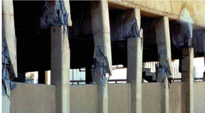
Figure 5-29: Damaged parking structure, Whittier Narrows (Los Angeles) earthquake, 1987. The deep spandrels create a strong-beam, weak-column condition.
