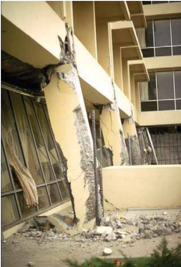
Figure 6-4: Sylmar, 1971, Damage to engineered building at Olive View Medical Center.
