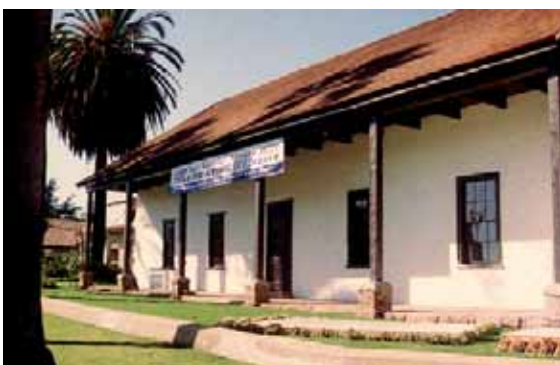
Figure 8-26: The museum at San Gabriel Mission, southern California, a historic adobe structure damaged by earthquakes in 1987 and 1994. It was repaired and strengthened, including installation of a bond beam of steel in the attic, anchor bolts into the wall, and stitching of cracks back together on the interior walls.
