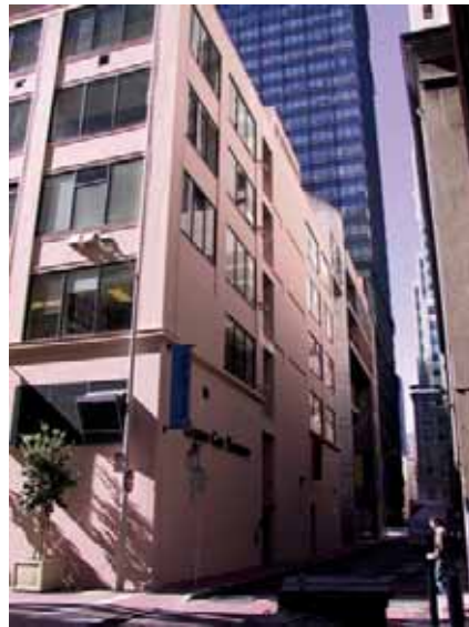
Figure 8-18: Infill of certain panels of an exterior wall for strengthening. Originally on the alley wall, only the central stair tower was solid wall, and elsewhere the upper window panel pattern was typical to the street.
