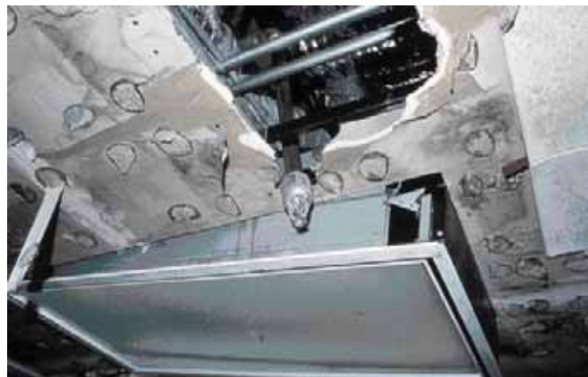
Figure 9-7 Example of systems interaction failure.
