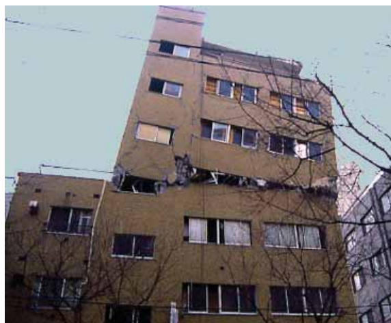
Figure 5-30 Damaged building, Kobe earthquake, Japan, 1995.
