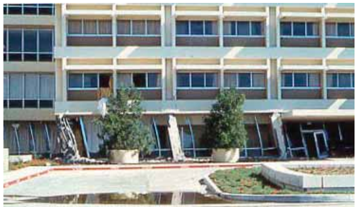
Figure 5-15: Olive View hospital, San Fernando earthquake, 1971, showing the extreme deformation of the columns above the plaza level.
