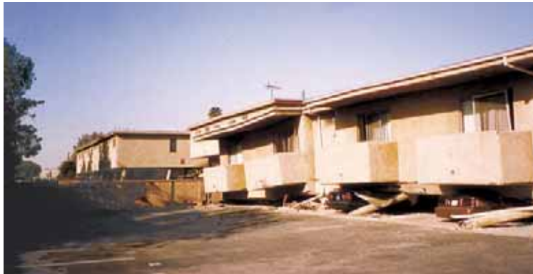
Figure 8-4: A 1970s building type with a deficiency not prohibited by the code at the time—a tuck-under apartment with parking at the ground level, creating a weak story. Many of these buildings collapsed in the Northridge earthquake. Sixteen deaths occurred in the Northridge Meadows apartments, or 42% of those directly killed by the earthquake.
