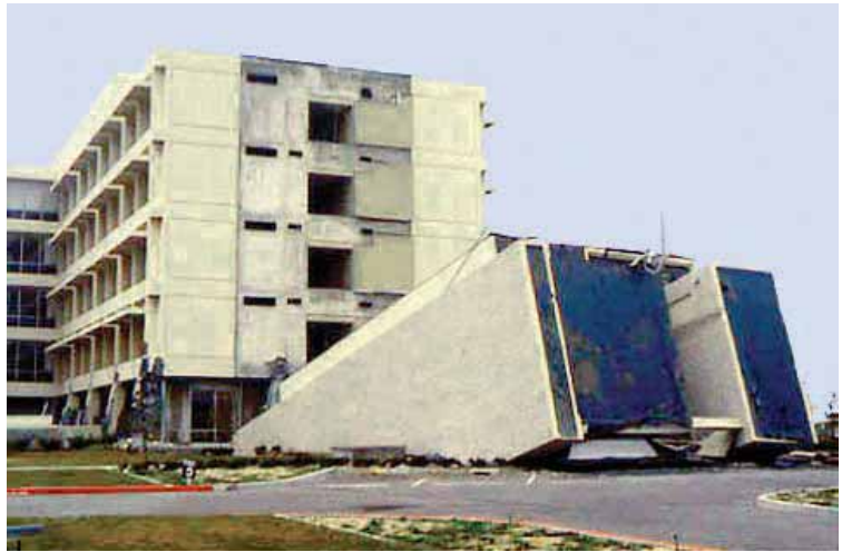
Figure 8-2: Olive View Hospital. A brand new facility that was damaged beyond repair in the 1971 San Fernando earthquake due to a shaking intensity that exceeded what was expected at the site and a design that, although technically complying with code at the time, contained several structural characteristics now considered major deficiencies. The lateral system contained nonductile concrete frames, discontinuous shear walls, and a significant weak story.
