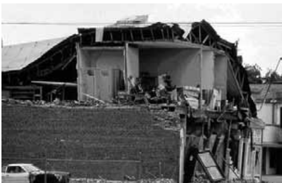
Figure 9-4: Nonstructural partition walls prevented the total collapse of this unreinforced masonry structure in the 1983 Coalinga earthquake.
