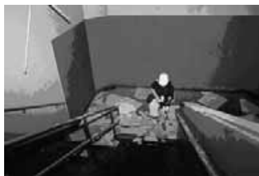
Figure 9-6: Difficulty in exiting due to debris strewn across exit stairs can be an indirect threat to life, as can be seen in this photo following the Loma Prieta earthquake in 1989.
