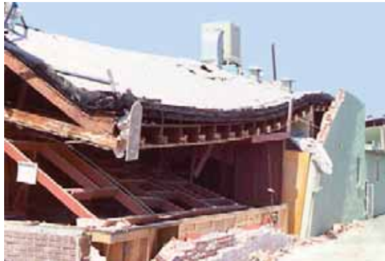
Figure 8-1: Example of buildings with no code design. Damage shows classic URM deficiencies.
