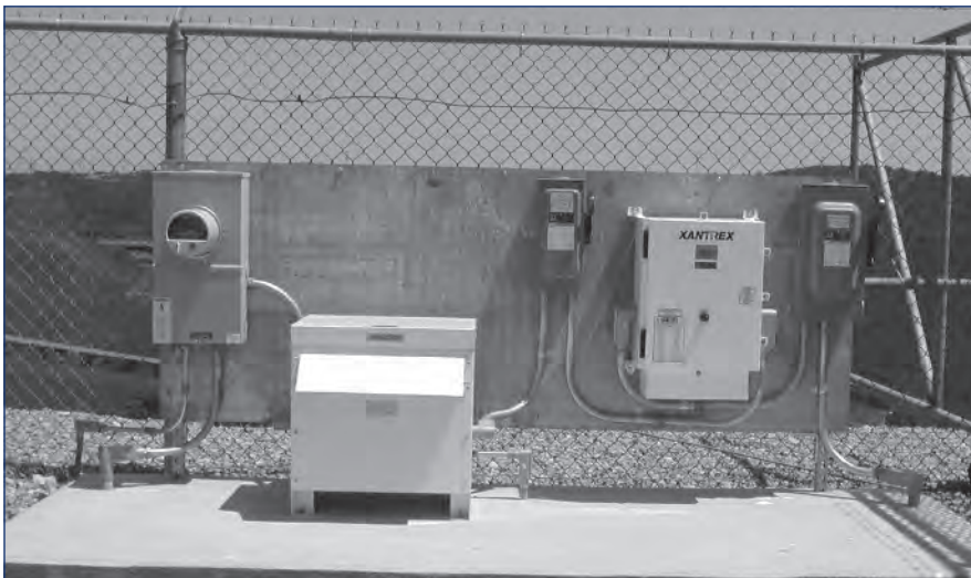
Figure 3. Balance of system components, including switchgear and inverter.
