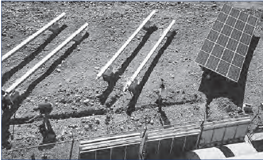
Figure 4. Aerial view of mounting structure showing I-Beams on concrete footings.
