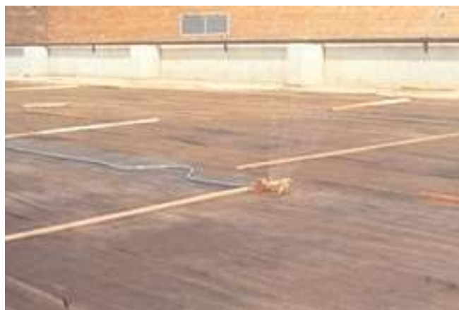
Fig. 12-5. Lawn sprinklers saturating burlap with water keep the concrete continuously moist. Intermittent sprinkling is acceptable if no drying of the concrete surface occurs. (50177)
