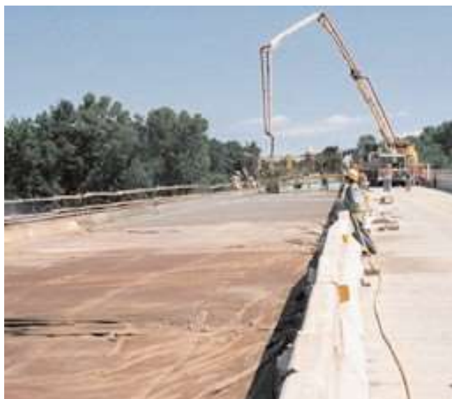
Fig. 12-1. Curing should begin as soon as the concrete stiffens enough to prevent marring or erosion of the surface. Burlap sprayed with water is an effective method for moist curing. (69973)
