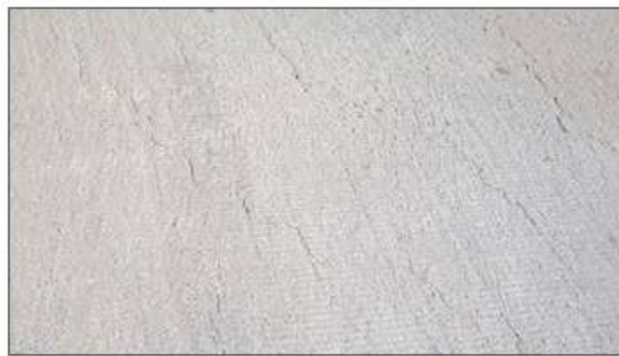
Figure 1. Example of plastic shrinkage cracking. Note, the closely spaced, parallel cracking
