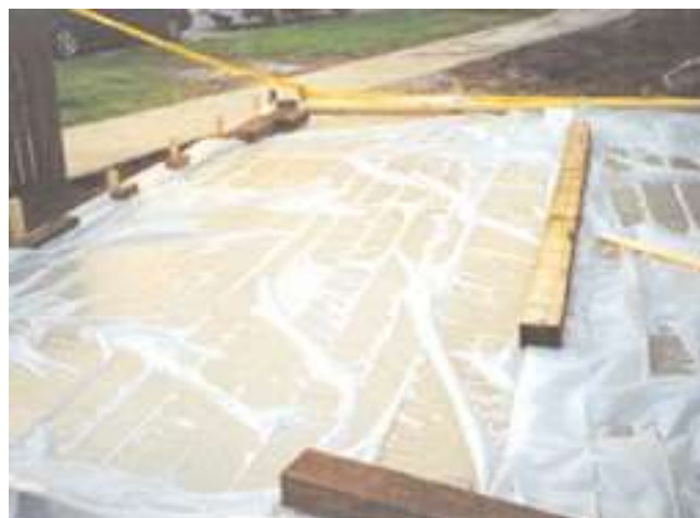
Fig. 12-7. Polyethylene film is an effective moisture barrier for curing concrete and easily applied to complex as well as simple shapes. To minimize discoloration, the film should be kept as flat as possible on the concrete surface. (70014)
