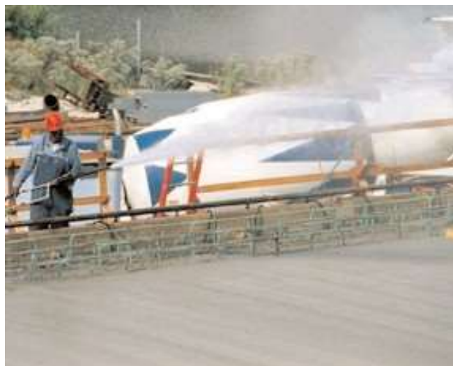
Fig. 12-4. Fogging minimizes moisture loss during and after placing and finishing of concrete. (69974)
