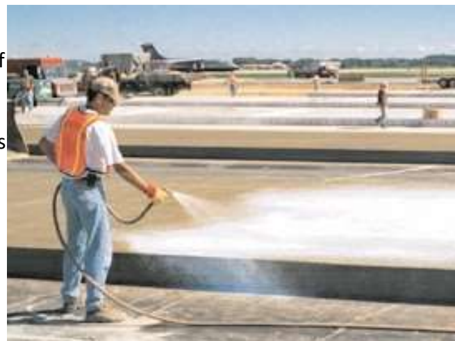
Fig. 12-8. Liquid membrane-forming curing compounds should be applied with uniform and adequate coverage over the entire surface and edges for effective, extended curing of concrete. (69975)
