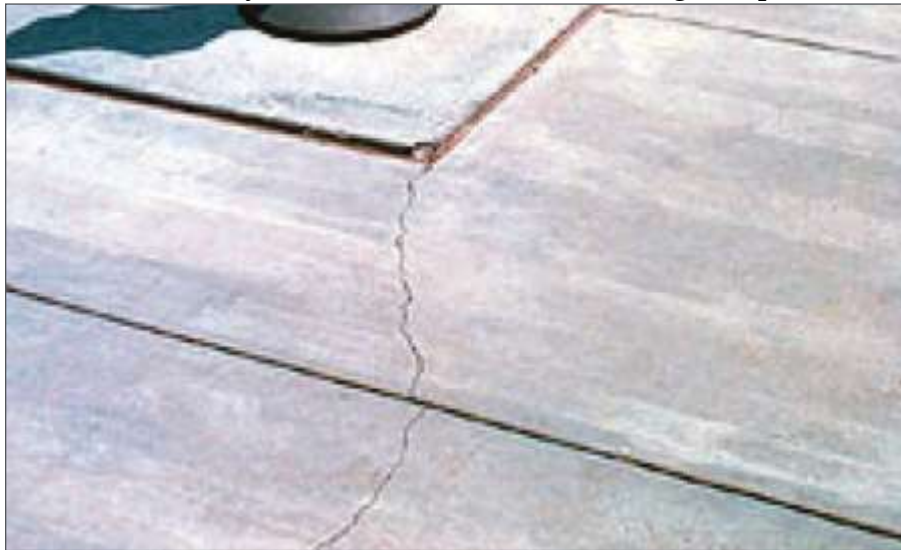
Figure 3. Drying Shrinkage Cracking.
