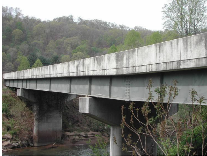
Figure 14. Photo. Bridge in West Virginia with a single-coat inorganic zinc-rich paint system after 25 years.
