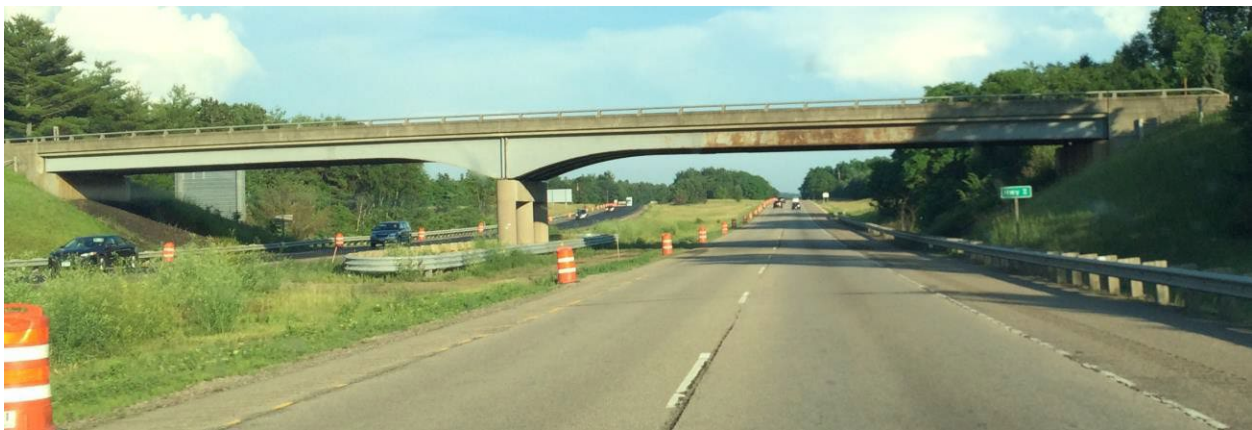
Figure 26. Photo. Accelerated corrosion on the inbound fascia girder of a grade separate structure, particularly over the right travel lane.
