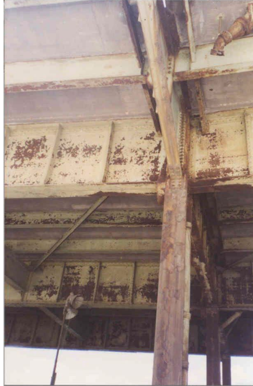
Figure 21. Photo. Missing portion of deck drain downspout.
