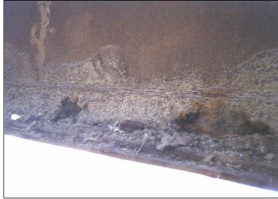
Figure 28. Photo. Heavy corrosion of bottom flange and web due to collection of poulitice.
