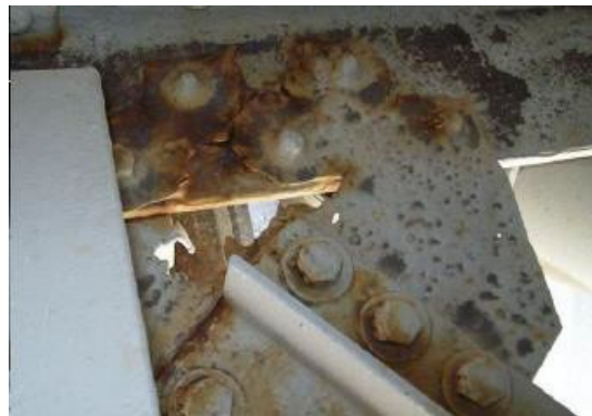
Figure 38. Photo. Corroded lateral gusset plate detail.
