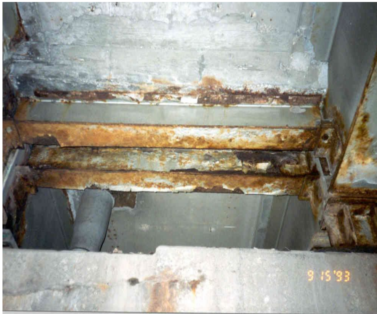
Figure 16. Photo. Steel directly beneath transverse expansion joints that have leaked corrosive runoff from the deck.
