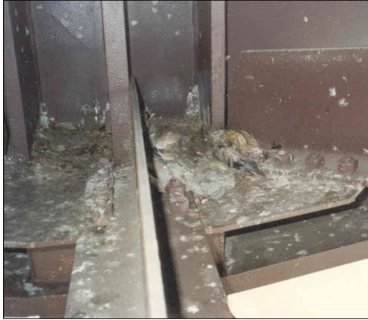
Figure 37. Photo. Debris accumulation at a lateral gusset plate detail.
