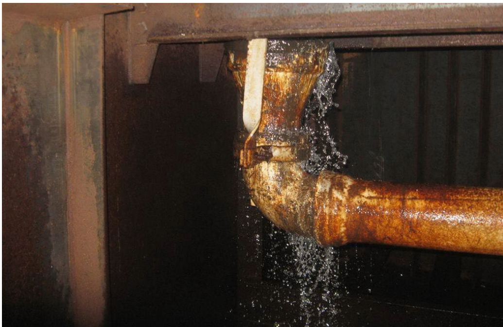
Figure 22. Photo. Clogged drain leaking water onto superstructure.
