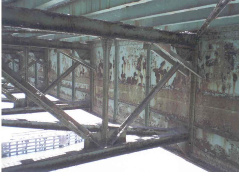
Figure 20. Photo. The area under an open grid deck acting as one large leaking joint.
