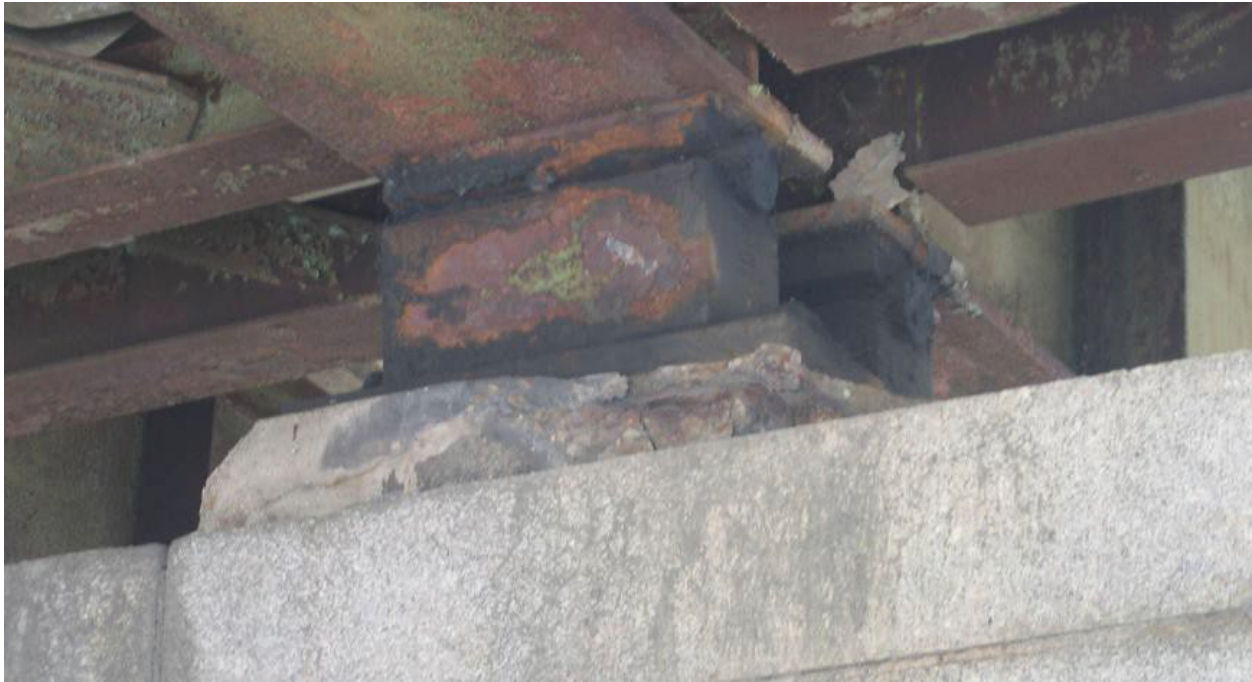
Figure 30. Photo. Corroded bearing.
