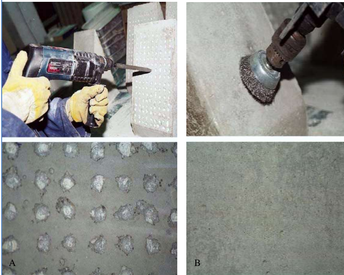
Figure 3.2. A) Substrate surface partially chipped, B) Substrate surface prepared with steel brush (Julio et al., 2004)
