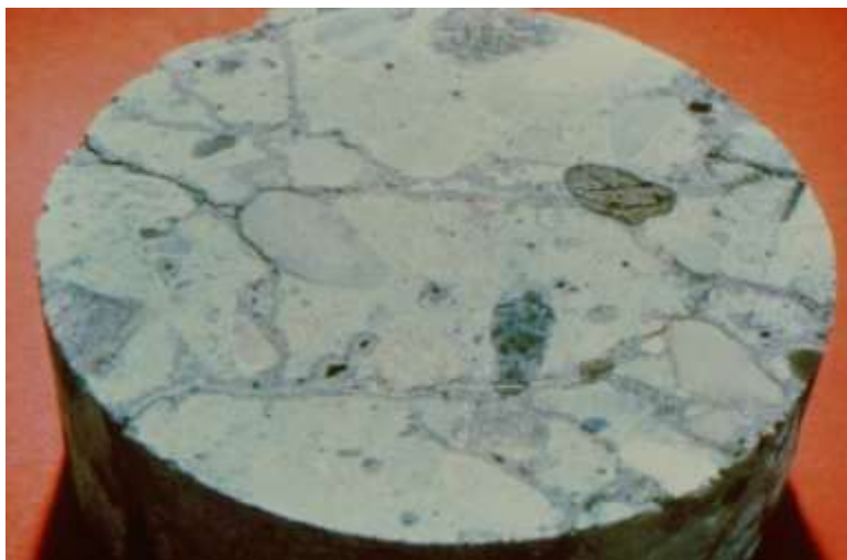
Figure 2.2. Cracks caused from ASR reaction (Glenn Smoak, 2002)
