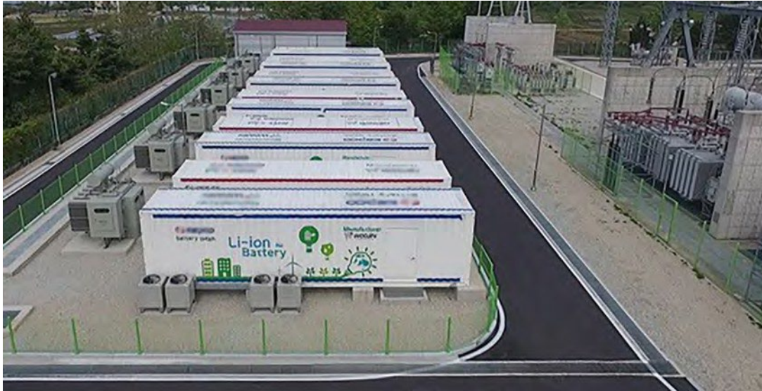
Figure D.4: Sokcho Battery Energy Storage System
