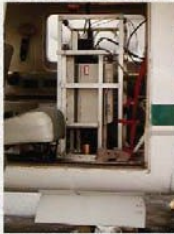
Transceiver installs in mid-body section of the Partenavia Explorer (Aspen Helicopter Inc.)
