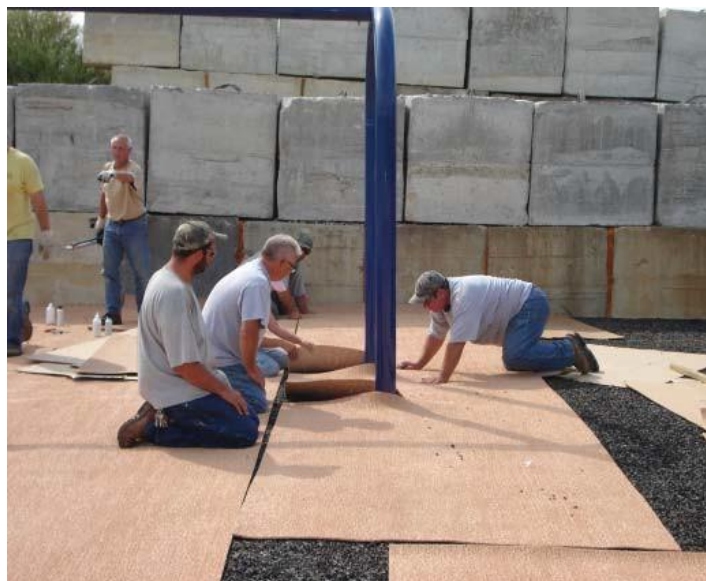
The base layer of crumb rubber has been installed. The top layer, a rubber mat system, is fit around equipment and the seams are joined. Both the equipment and surface system at this site will be installed by the park maintenance crew.
