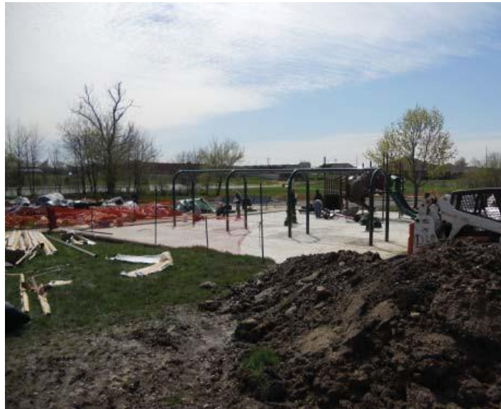
The playground site has been graded with earth-moving equipment. The concrete base has been prepared and is awaiting the application of the poured-in-place rubber (PIP) system. At this site, the playground equipment and surface system will be installed by a contractor specializing in playground construction.
