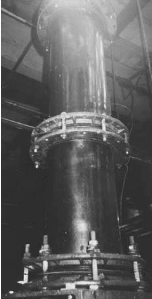
Figure 8: Glass Section of 8-inch Line to Condenser
