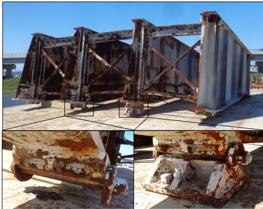
Figure 29 – South girder bearings after the incident
