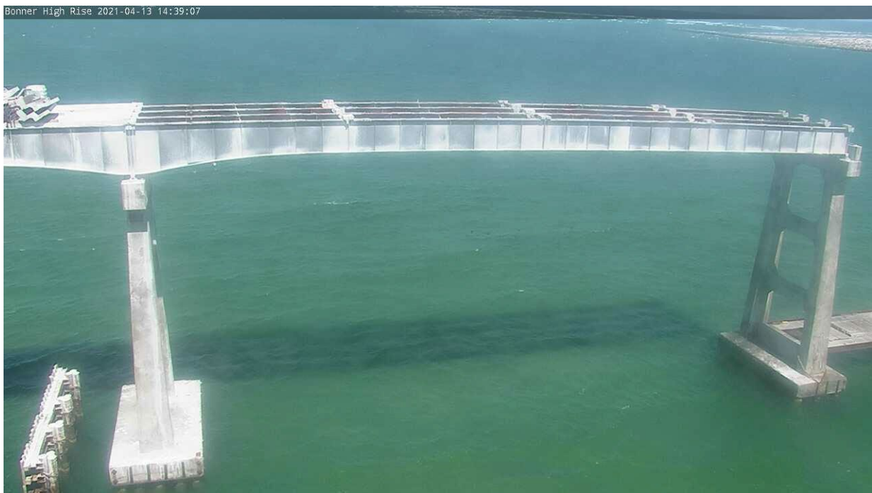
Figure 24 – Concrete in Span 146 had been removed (photographed on 4/13/2021 by NCDOT)
