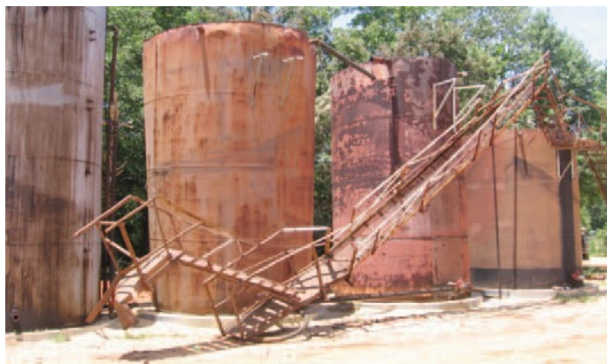
Tanks involved in the 2006 accident that killed three workers at the Partridge-Raleigh Oilfield.
